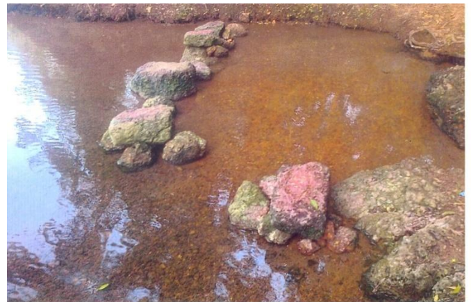
Completion of work undertaken on desilting of lake at Harizanwada of V.P. Advalpal.
