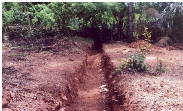
Final stage of construction of kutchra gutter from Shigao market to river point Via Narshiv Naik agriculture farm, in V.P. Collem under MGNREGA Scheme.
