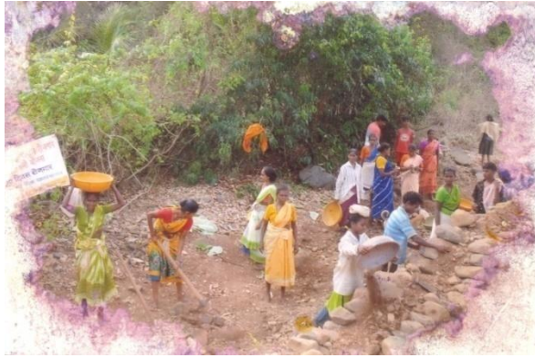
Job card holders at work during construction of Nallh Bank Pitching (flood control) at waizawada in v. p Shristhal
